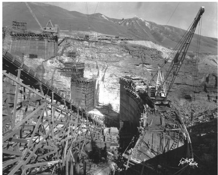
Kerr Dam under construction, 1937. Photo: C. Owen Smithers, courtesy Smithers & Son Photography, Butte, MT.
