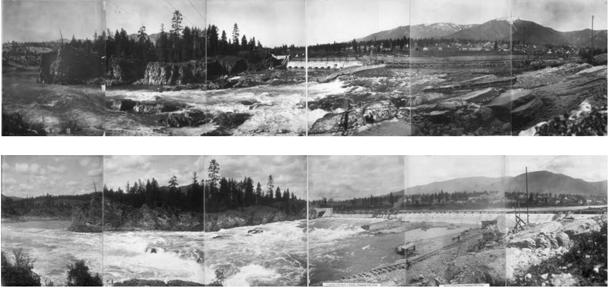
Top: Thompson Falls Dam under construction, 1914. Above: the completed dam, 1915. Library of Congress.
